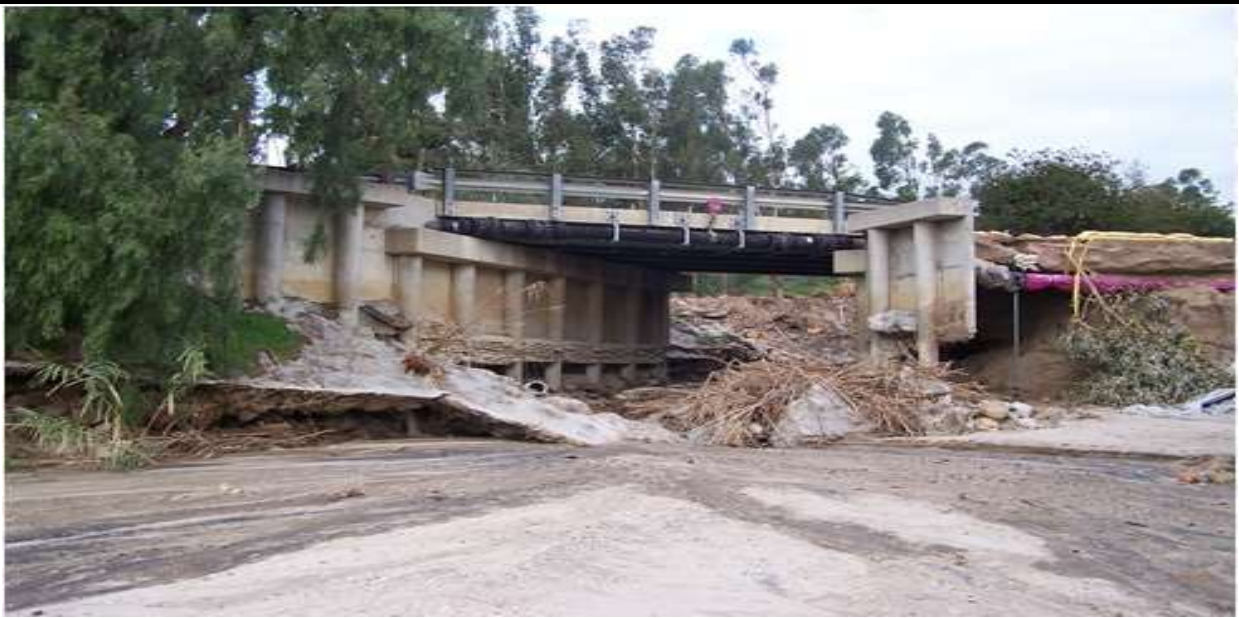
Figure 5: Structural integrity near hydro geological site and poor soil condition
